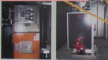
Hogged wood heating station (550kW) and peak load boiler (1600kW)
