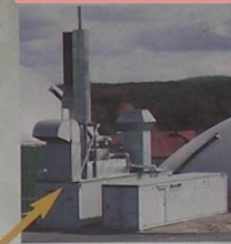
Block-heat power station (700kW el ) and pump container
